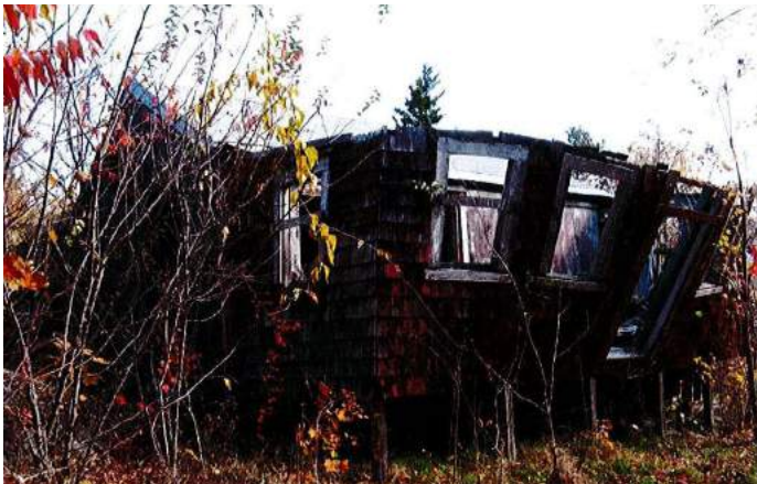
Collapsed front porch, Cottage 38.
