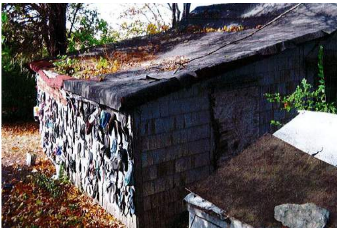
SE view of Cottage 30 showing roof condition.
