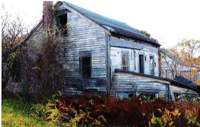
Collapsed front porch to Cottage 21.
