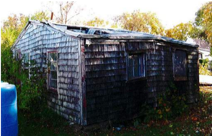
Collapsed roof, Cottage 39.
