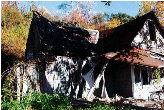
Deteriorated state of Cottage 46.
