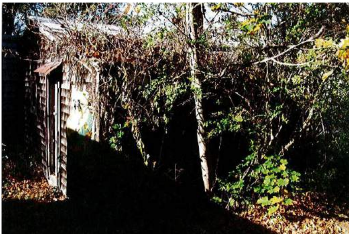
Overgrown condition of Cottage 39, SE corner.
